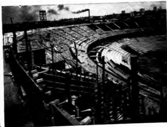
1, the gymnasium under construction. 2, model and section of the gymnasium and perspective of the completed group.
